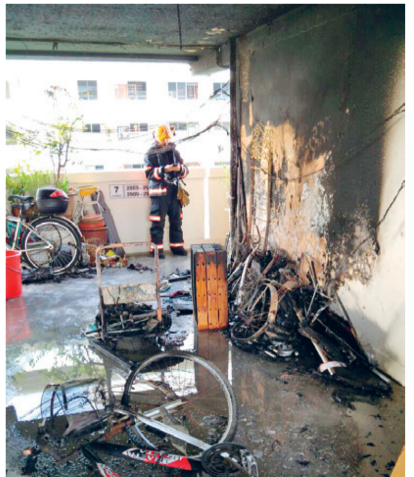
7 April 2016: fire involved items placed at the corridor in Eunus Crescent.
